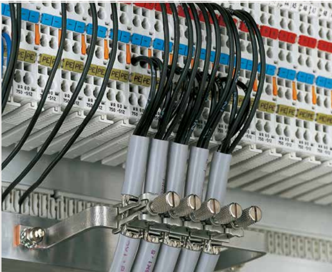
U-shaped (10 x 3) mm copper busbar
